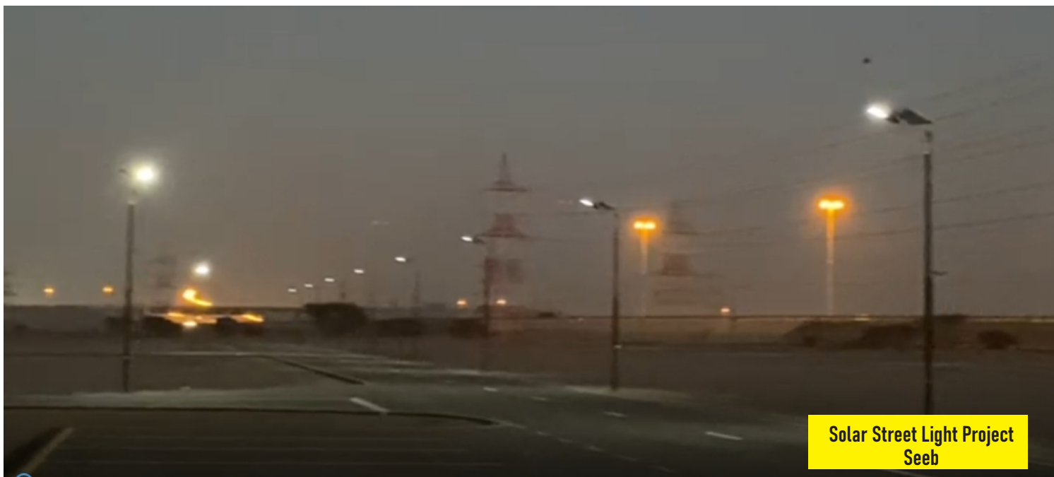
Solar Street Light Project Barka - Naseem Garden
