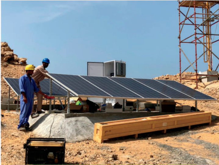
Solar off-grid system, PDO (Oman)
