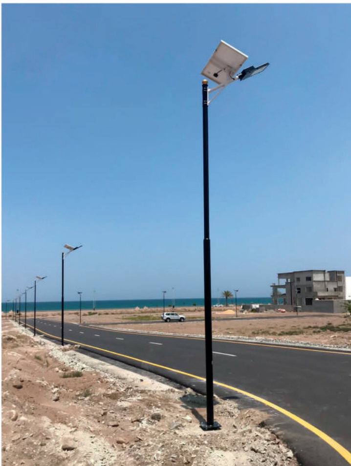
Solar Street Lights, Al Hail
