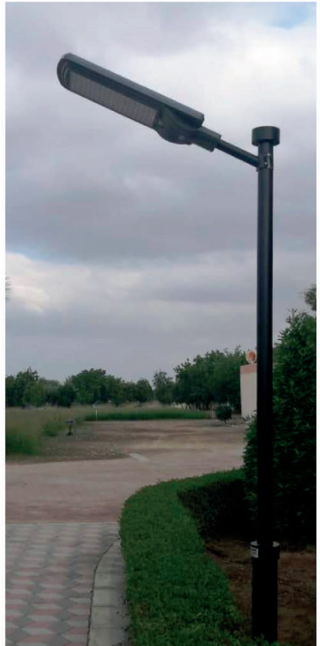
Solar Street Lights, Al Mouj
