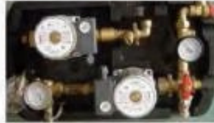
Include Wilo RS15/6 pump station, SP618 controller, water flow meter, water pressure meter, expansion tank, safety valve
